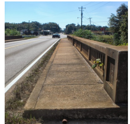
Narrow bridge over railroad tracks on SC Highway 81 between Blue Hole and downtown.
