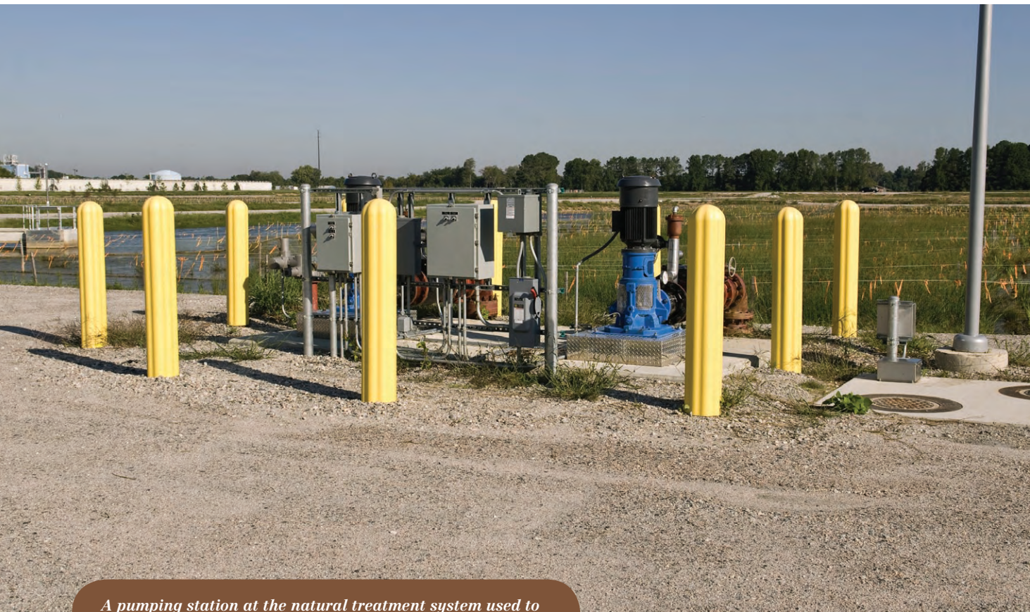
A pumping station at the natural treatment system used to pump effluent as needed during high flows.
